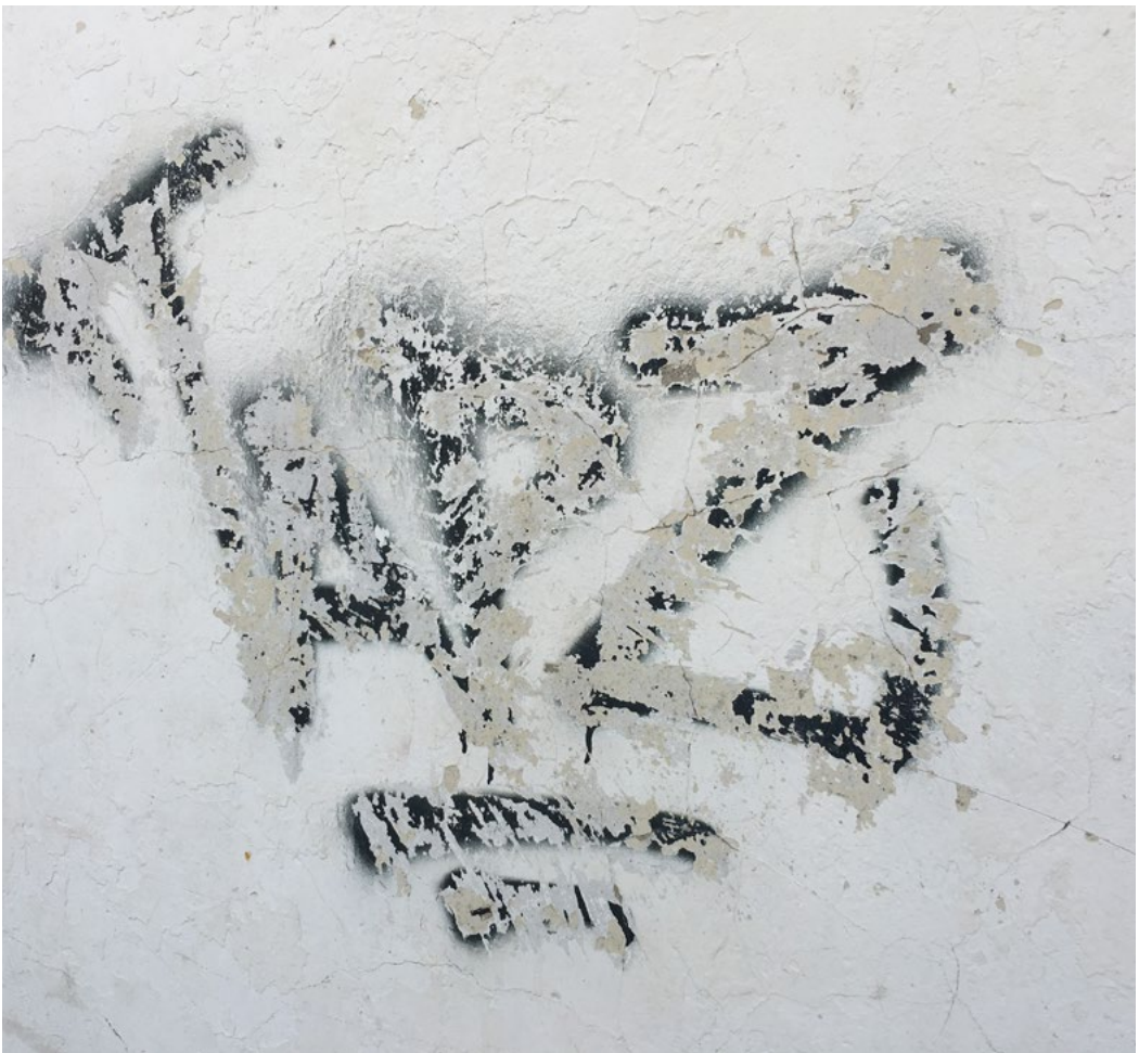
Figure 8: An unsuccessful attempt at the removal of a tag (January 2018). The painted surface has absorbed the spray paint.
