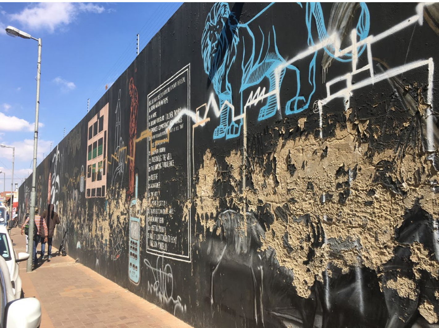
Figure 5: Flaking walls (August 2017). The medium of the work or the surface may also have limited longevity and so either the paint fades or the surface crumbles.
